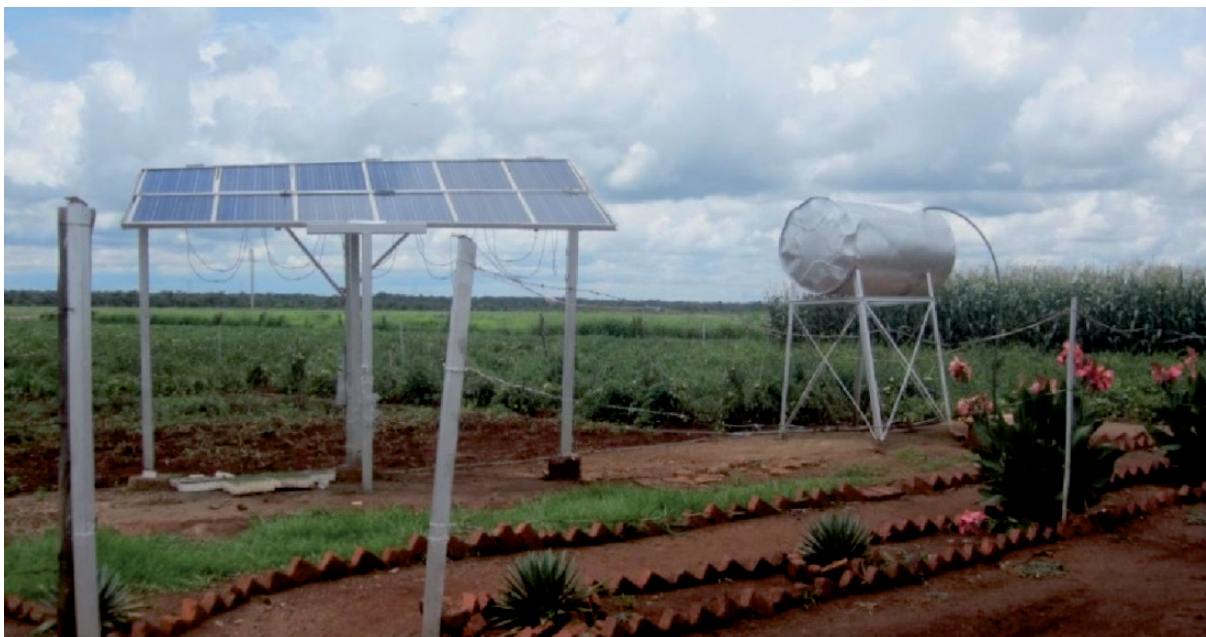
Figure 11.6 Solar-powered drip-irrigation demonstration
